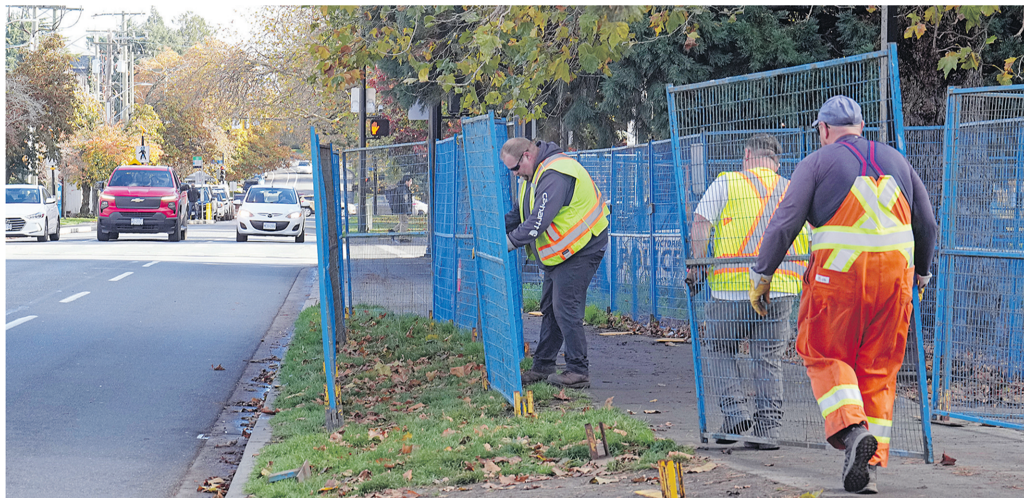
Victoria workers install fencing around the tented area in front of Our Place on Pandora Avenue. The fencing has cost about $10,000. ADRIAN LAM, TIMES COLONIST
